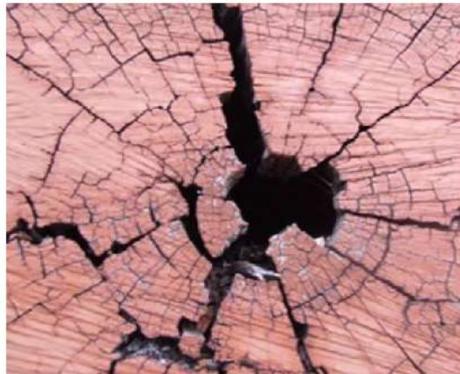
Plate 4.4 Cavity at the end of a rotted girder
