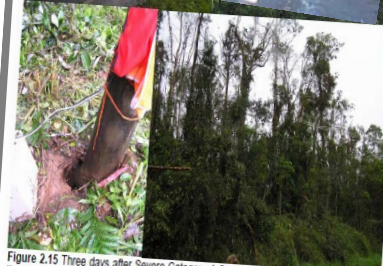
Figure 2.15 Three days after Severe Category 4 Cyclone Larry passed almost directly over the Palmerston Highway and the canopy bridges, showing canopy bridges still in place, slight sagging of the rope tunnel, pole shaken in ground and damage next to one of the ladders. Photos: S. Goosen
