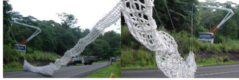
Figure 2.10 Ergon Energy cherry picker used to thread tunnel into position from electricity pole to tree support. Photos: Birgit Kuehn
